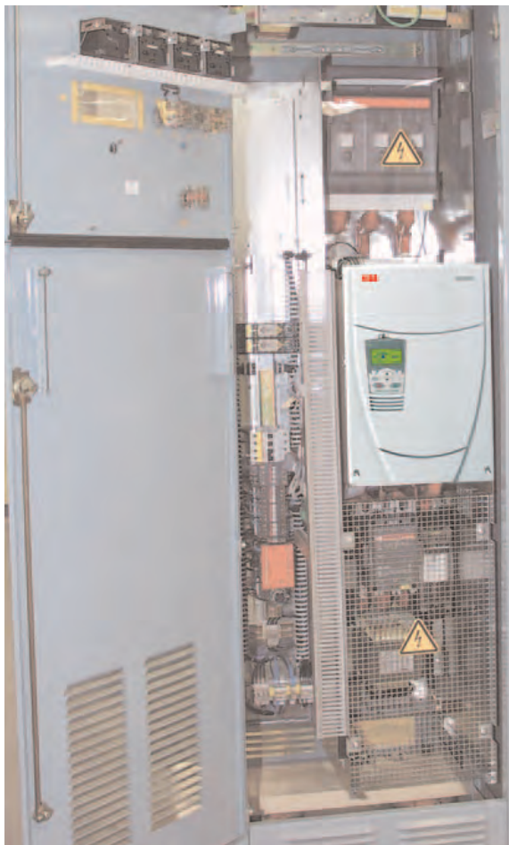
DCS800-E mounted in old cabinet
