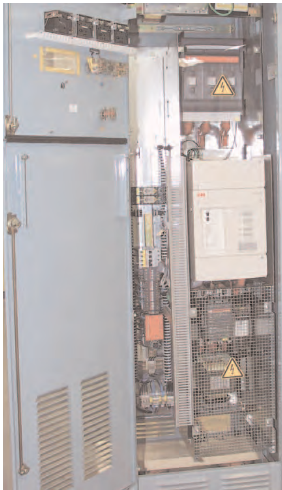
DCE mounted in old cabinet
